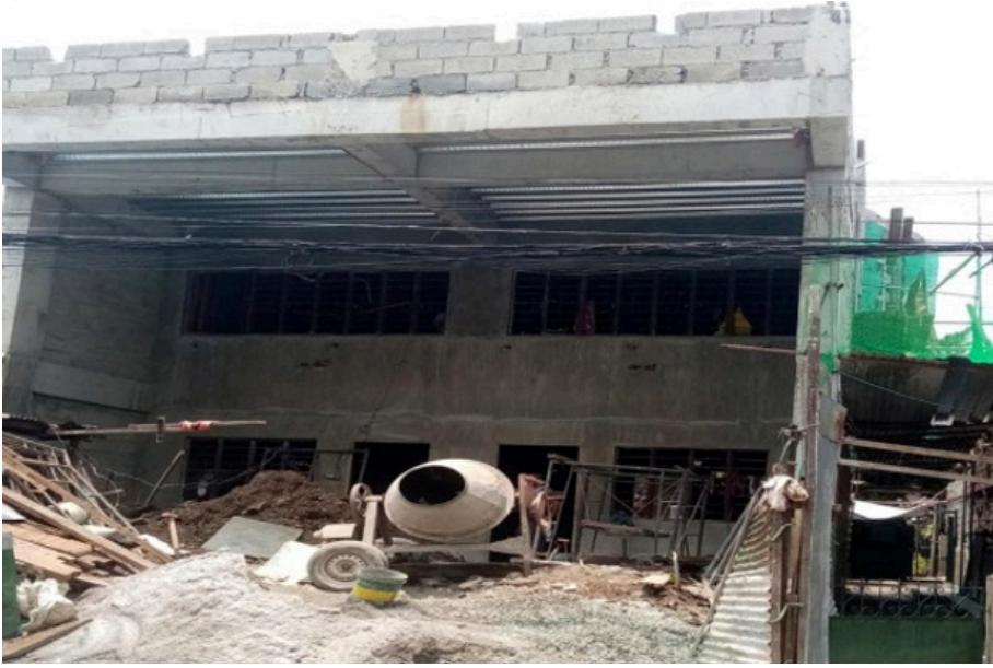
The lower and upper ground floors of the REACH headquarters are completed with a rough finish.
